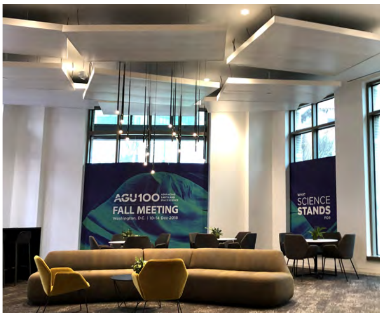
Picture 3. Radiant cooling panels in the lobby.
