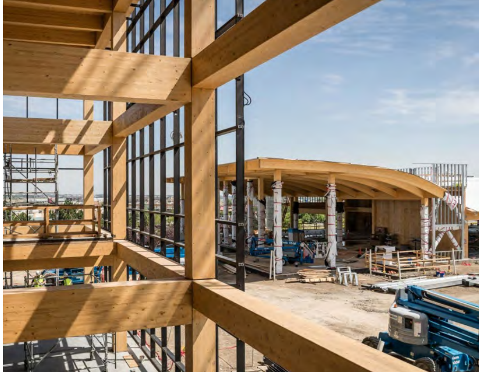
(Top) Sample Construction. Photo: Swinerton. (Bottom) Sample Modern Mass Timber Building. Photo: 25 King in Brisbane, Australia.
