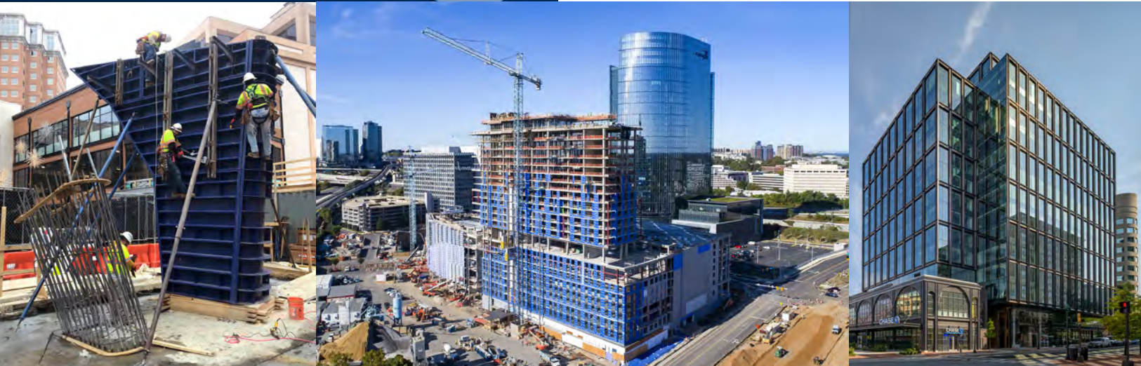
(Left to Right) Ballston Quarter Retail Renovation, Arlington, VA – Christman Mid-Atlantic Constructors, Inc.; Capital One Center – Miller & Long Co., Inc.; 4747 Bethesda Ave., Bethesda, MD – Ferguson Neudorf Glass
