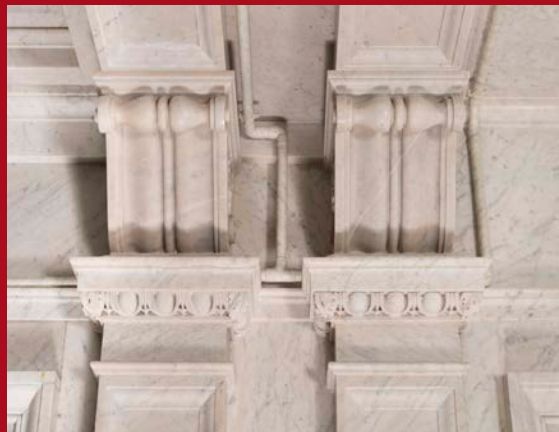
Winners for Visual Excellence The Thomas Jefferson Building Sprinkler System, West Main Pavilion, First Floor
