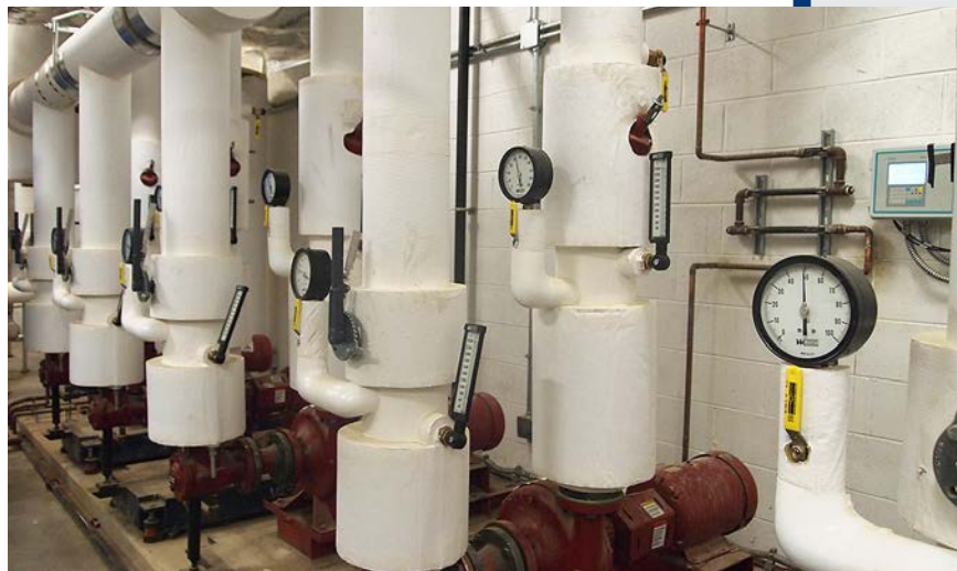
Mechanical: HVAC-Piping American University Washington College of Law, Washington, DC
