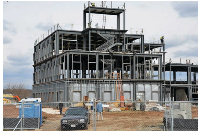
Costello Construction "Tops Out" Steel Construction of New $11-Million Building for Md. Air National Guard
