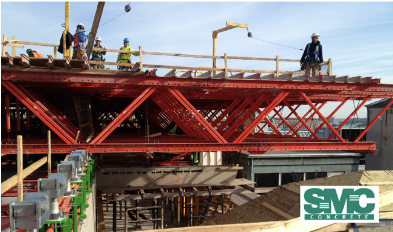
1700 New York Avenue - 33 ft cantilevered slab over glass roof of Corcoran Gallery of Art
