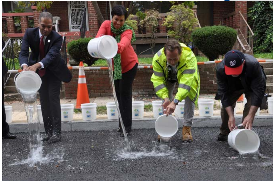
Attendees at the kickoff event showcase the performance of the newly installed porous asphalt. (From left to right: Councilmember Brandon Todd, Mayor Muriel Bowser, DC Water's General Manager and CEO George Hawkins, and DC Water Board Member Anthony Giancola)
