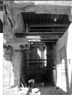
Above: St. Albans' new building, Marriott Hall. Left: A 35-foot underpinning pit at the St. Albans' construction site.
