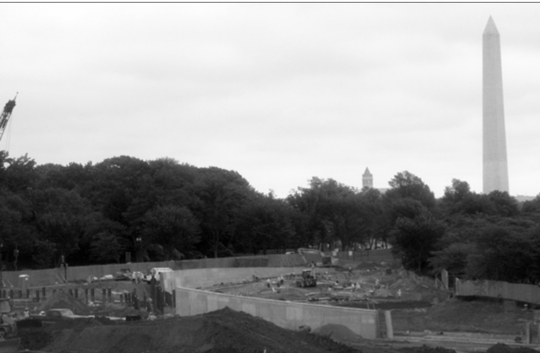
MTTG, the design/build joint venture team comprised of McKissack & McKissack, Turner Construction Company has begun work on the Martin Luther King Jr. Memorial.
